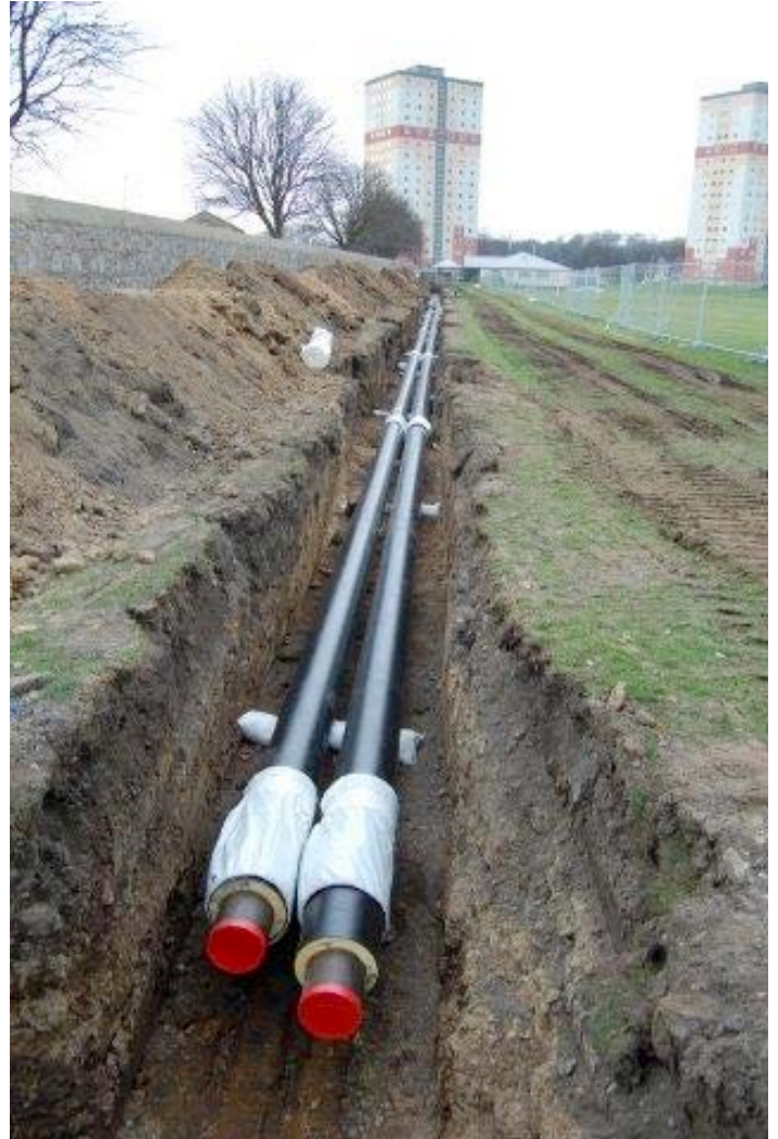
Image: Underground mains Seaton
